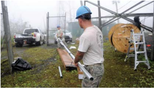
Installing an antenna on a communication tower in Puerto Rico (Source: FEMA 11/11/2017)
